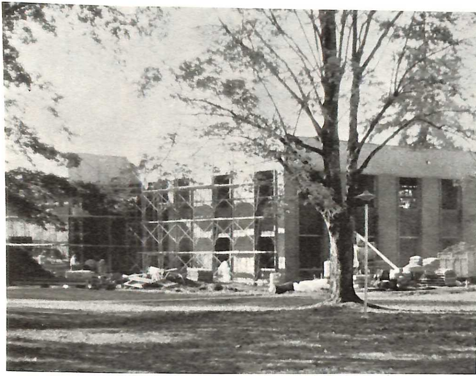
The new Herbert C. Hoover Academic Building is nearing exterior completion with masons placing final brick. The new $850,000 center, when completed early spring, will contain academic offices, classrooms, and the Kershner Center for Economics within the 20,000 square foot structure, south of Wood-Mar Hall.
