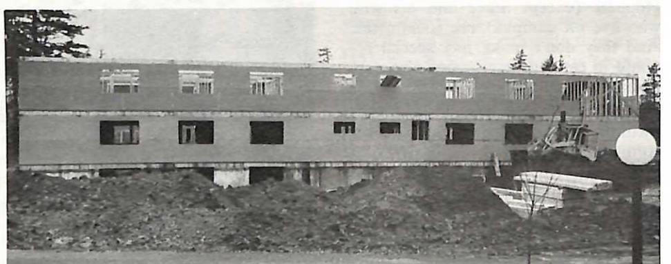
Workers for Bishop Construction Co. are on schedule with a $1.2 million project to complete a new student residential complex by September. Hobson Hall (in background) with 74 beds is the anchor unit for the complex that will house 202 students when completed. The two new three-story buildings will be similar in design to Hobson Hall and connected by underground and outside passageways.
