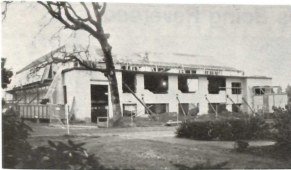
Workmen have begun the task of removing the old roof on the 30-year-old Hester Gym on campus as the building becomes the college's new Milo C. Ross Fine Arts Center in a $1.3 million project. Work crews removed the shingle roof, replacing the under structure in preparation for a new mansard roof. A new concrete first floor also has been poured, and the major supporting structure for a second floor is being placed.
