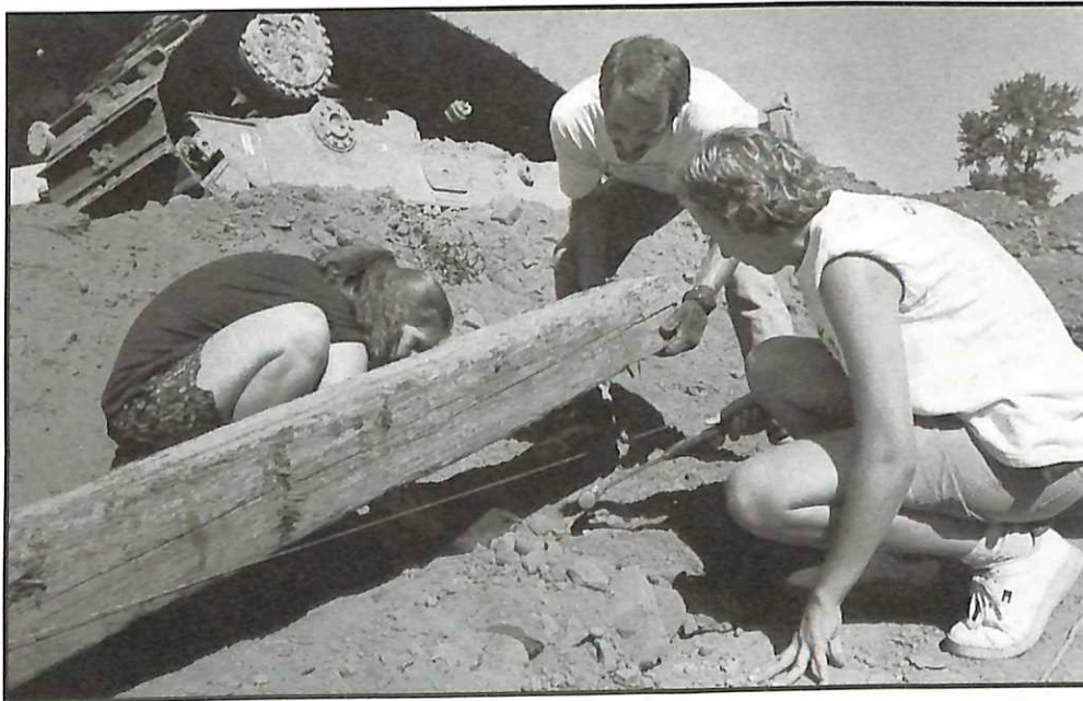
Sarah Powell, a sophomore from Turner, Ore.; Ron Mock, assistant professor of peace studies and political science; and Lauren Barnhart, a junior from Woodinville, Wash., (left to right) help construct a retaining wall for a new skateboarding facility at Ewing Young Park in Newberg.
