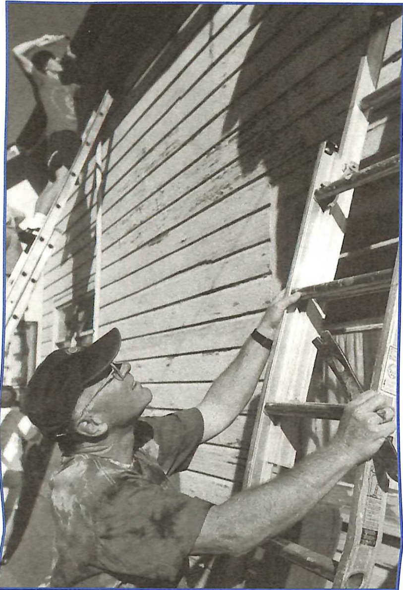
President Brandt steadies a ladder while serving on a work crew that prepared the house of Roy Hiebert, George Fox University's "campus grandpa," for a new coat of paint.
