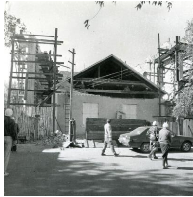
Prayer House of the First Community. Kyiv, Yamskaya, 70. Beginning of reconstruction (1994). The photo shows the old facade and the construction of new walls.
